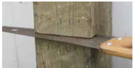
Photo 3a. Celtic framing technique. A hand saw makes a level cut 1.5 inches deep to provide bearing.
