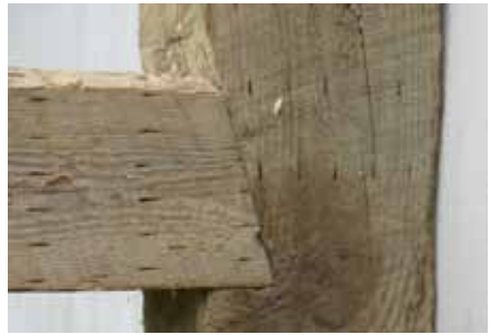
Photo 2. This mock-up shows how an angle-cut floor joist is notched into the face of a wall stud.
