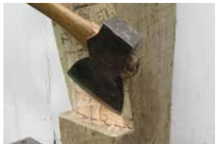
Photo 3b. Celtic framing technique, part two. The rest of the sloping notch is quickly cleared with a hatchet.
