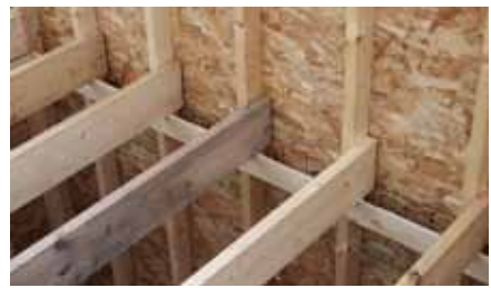
Photo 1. In balloon framing, second floor joists sit on a 1 inch by 4 inch board called a ribbon. (All photos by Bruce MacNab)
