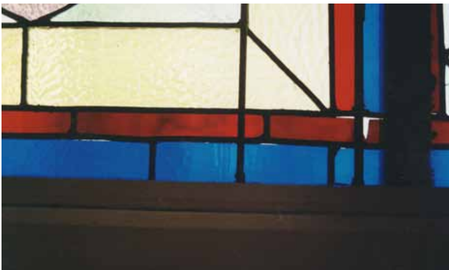
Glass separating from lead came.
