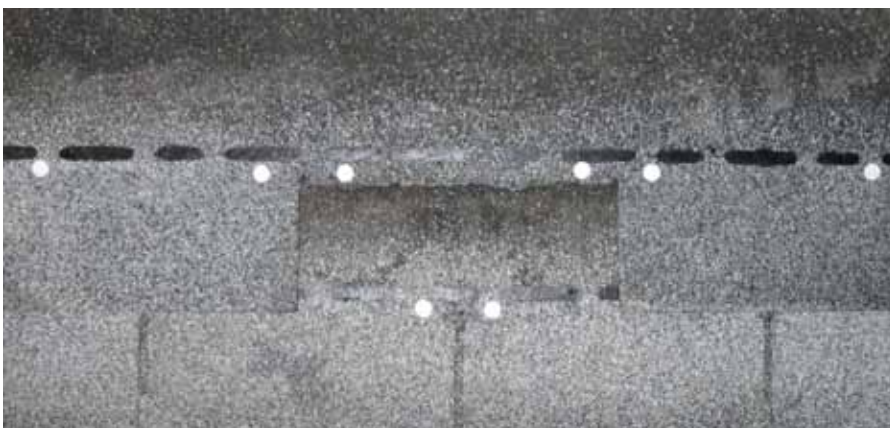
It's better to lose a tab (above) rather than the entire shingle. The six nail pattern used here is called storm-nailing. Note: Dimes used as nails. (Not recommended for installations!)
