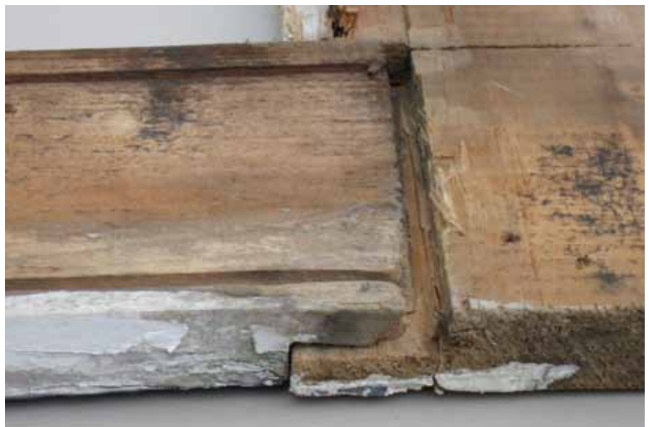
Photo 3: Back side of head-lap detail. This self-flashing joint was crafted with hand tools many years ago. Note: The vertical grooves diverted rain water in lieu of caulking.
