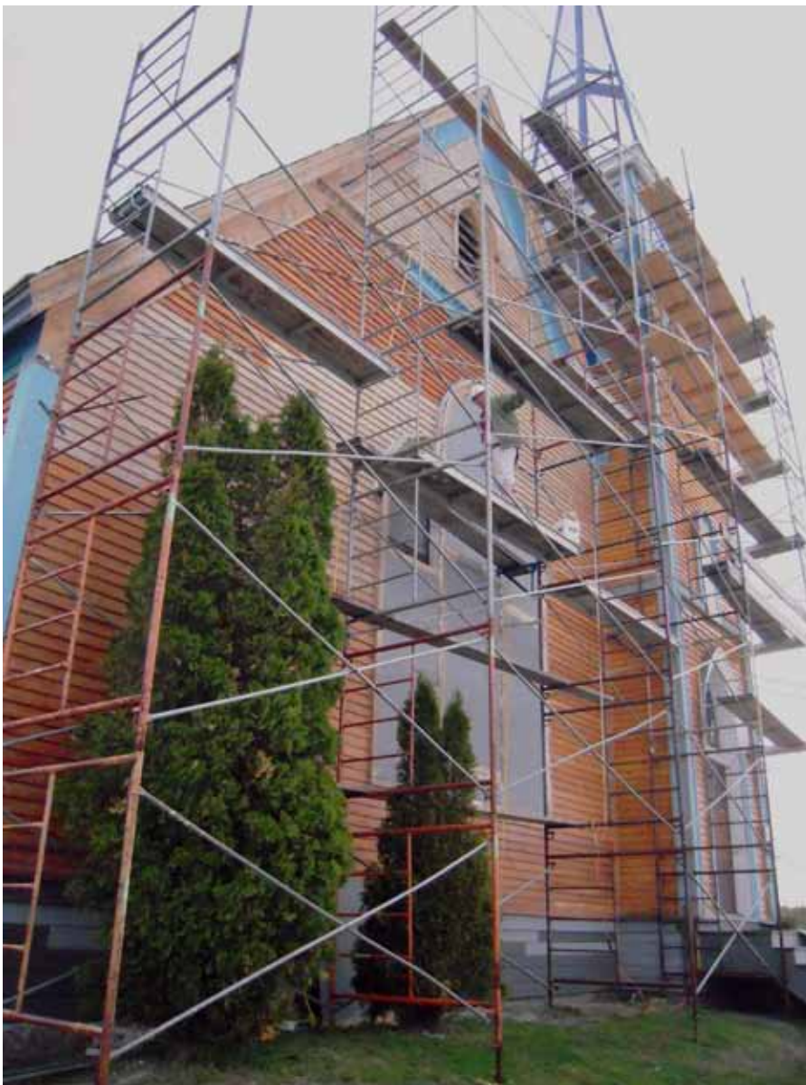
Lori Nason braving the elements and heights while working on the west windows.
