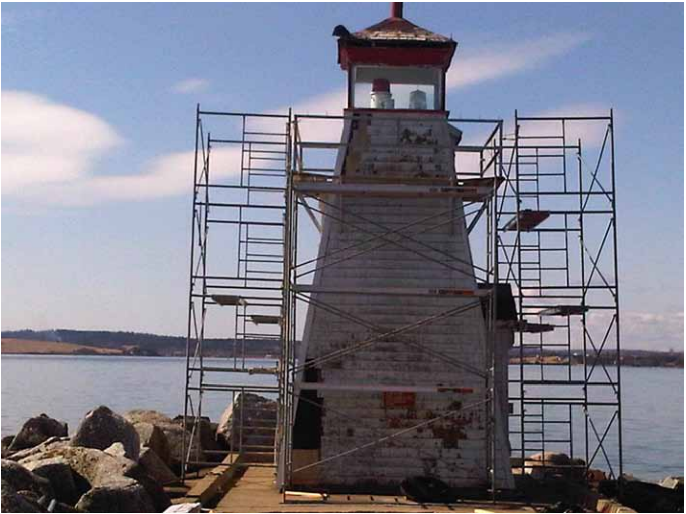
During 2010-11 students worked on the Battery Point Light in Lunenburg Harbour, a project completed under the supervision of instructor Paul MacLellan. (Courtesy of NSCC)
