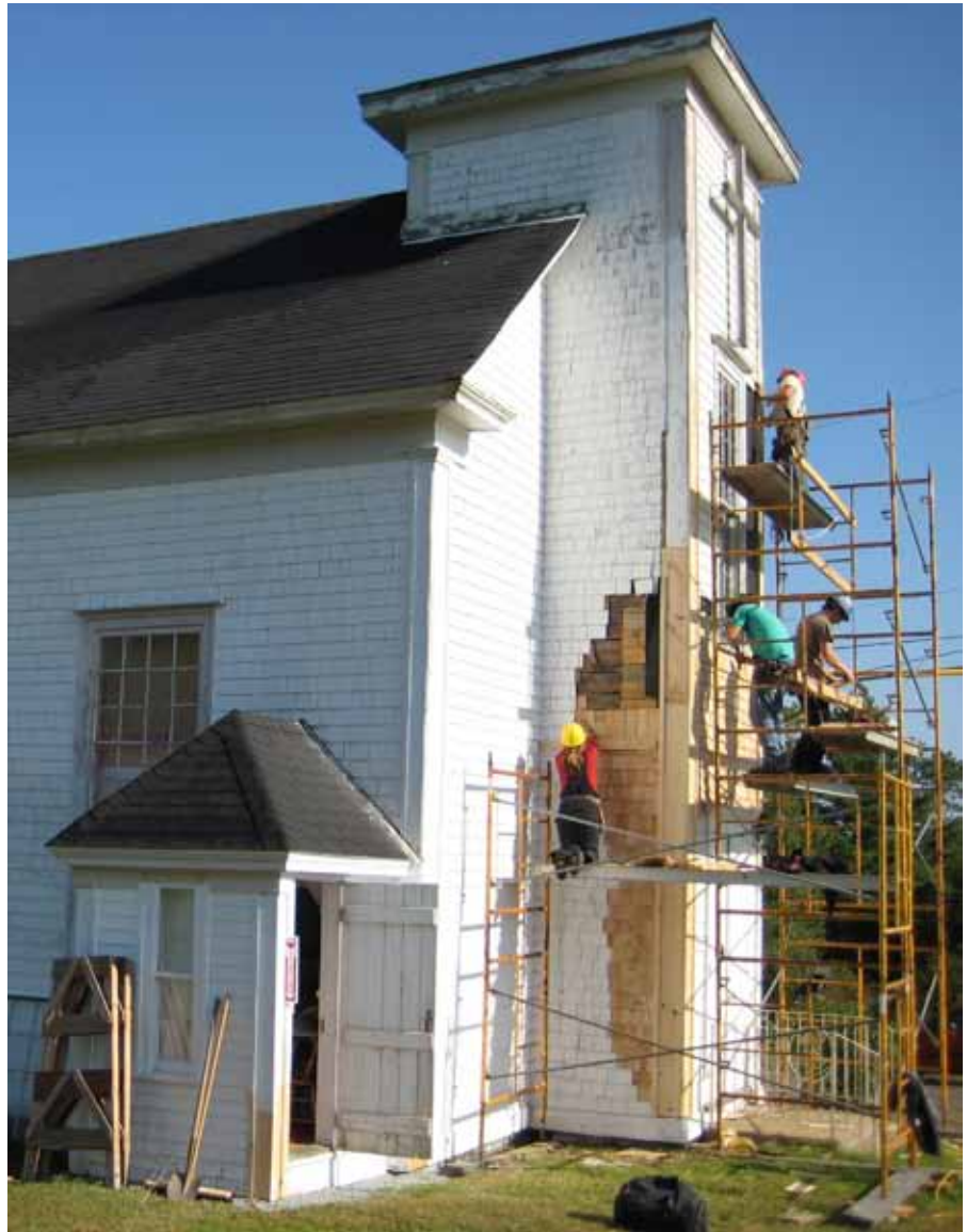
Work on Saint Mark's Evangelical Lutheran Church in New Cornwall was completed in 2009 by a class of second-year students. (Courtesy of NSCC)
