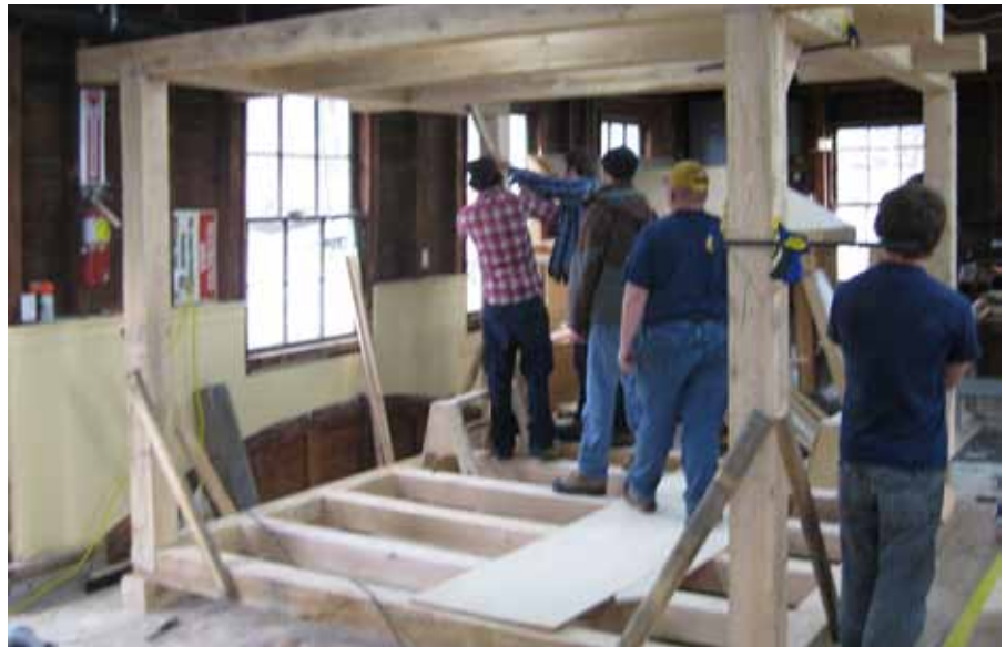
Students pre-assembling a timber-frame structure in the NSCC's Lunenburg shop. (Courtesy of NSCC)
